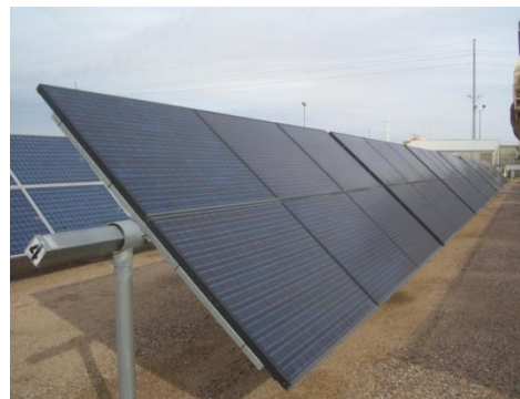
Figure 12. Photograph of OPV2B Modules
