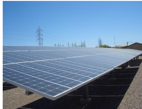
Figure 10. Photograph of OPV1B modules
